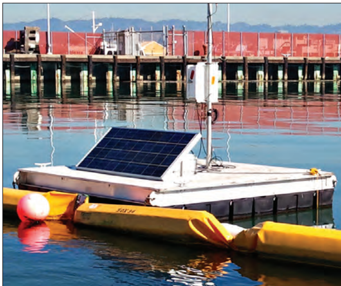
WQ-PAD deployed in San Francisco Bay.
